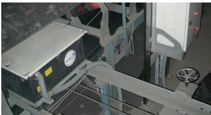
CNA 3 installed 800 m underground in the LKAB iron ore mine at Malmberget (Northern Sweden)
